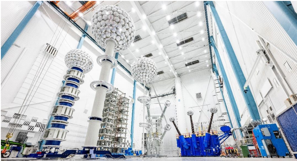
High-Voltage Direct Current (HVDC) power transformer testing area in one of Hitachi Energy's facilities in Europe
