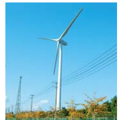
2,000 kW wind power generator developed jointly with Fuji Heavy Industries Ltd.
