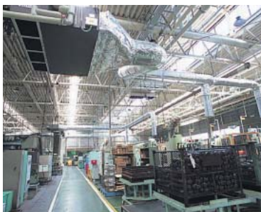
Displacement air conditioning equipment at Komatsu Ltd. Oyama plant
